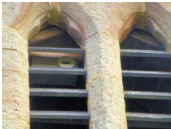
Fig 2: One of 4 swift boxes provided during the renovation works.
